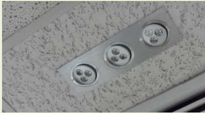
LED ceiling light in SP office
